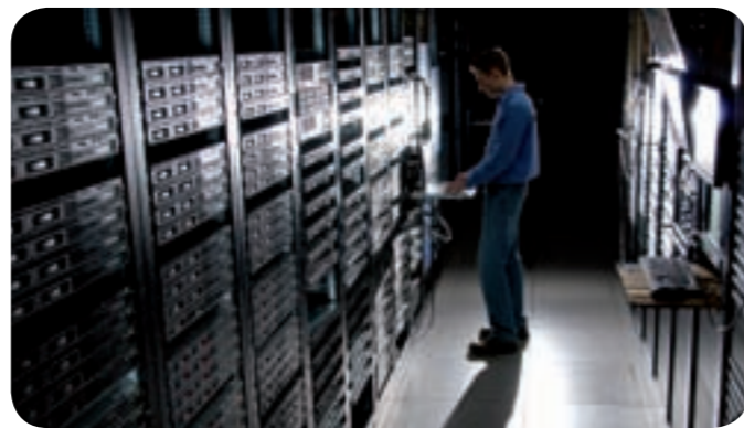
In the SPEED Broadcast Equipment Room, Dalet Enterprise Edition runs on standard IT servers and integrates with storage and broadcast systems.
